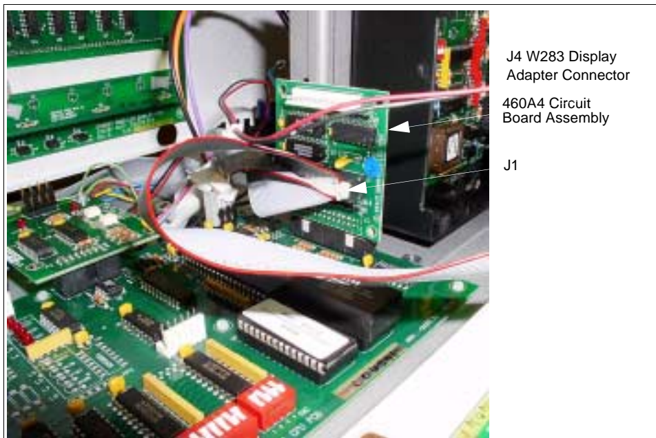
Figure 20: 460A4 Circuit Board in Place with Connections Made
